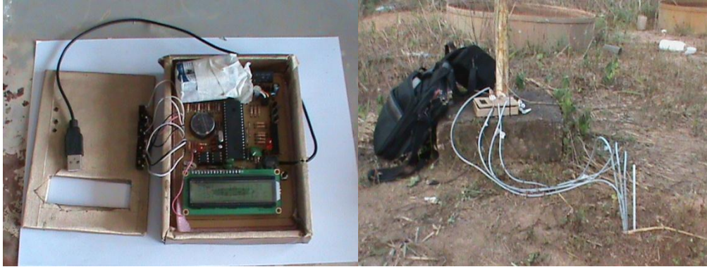
Plate 2: Fabricated datalogger and the TDR water sensor installed in the soil
